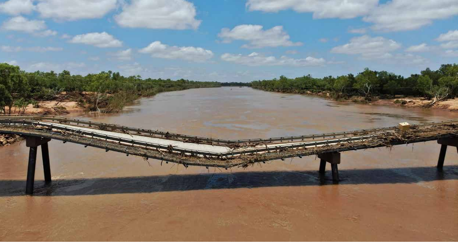
Flooding generated by Ex-Tropical Cyclone Ellie in December 2022 and January 2023 caused significant damage to the Fitzroy River Bridge. Credit: Main Roads
